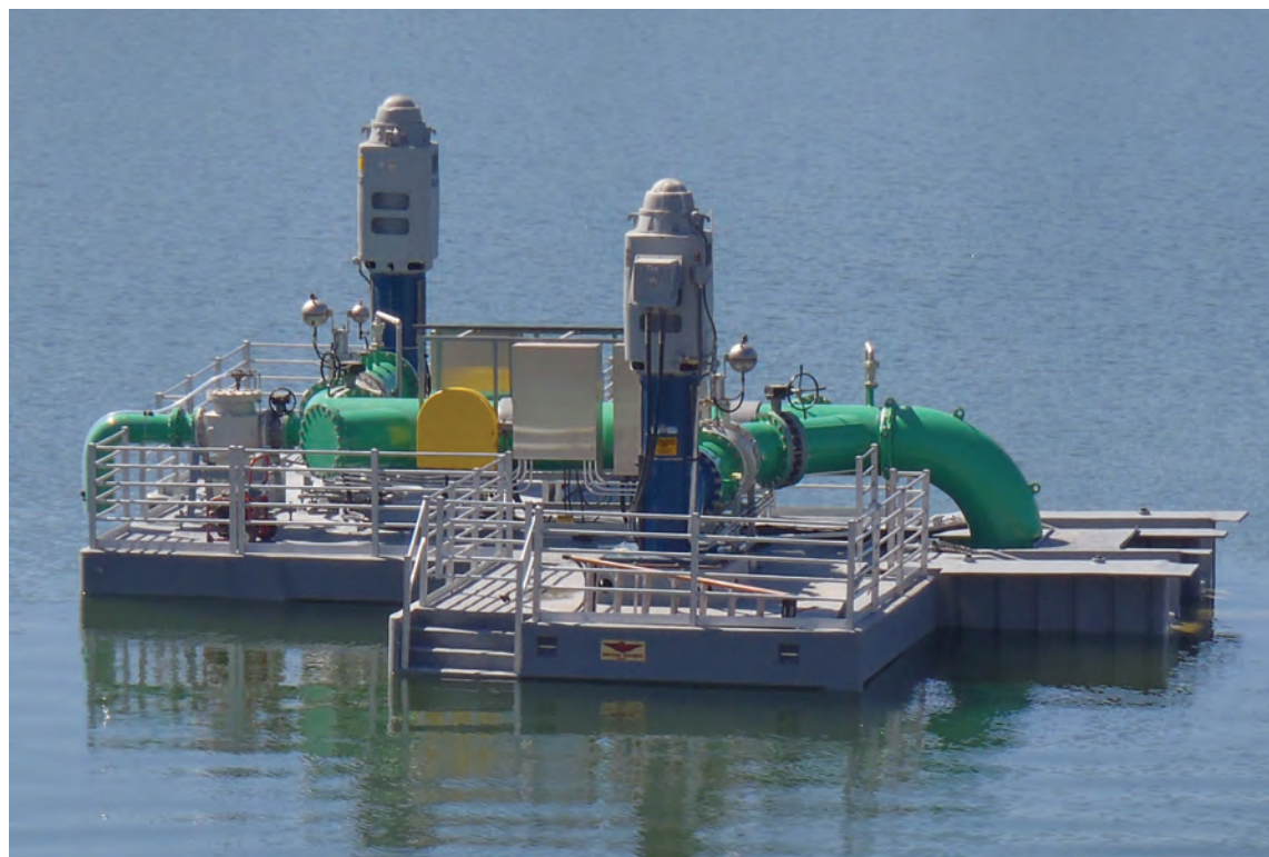
The floating pump station allows for the transfer of stored water from OCWD's Santiago Basins to other OCWD facilities.
