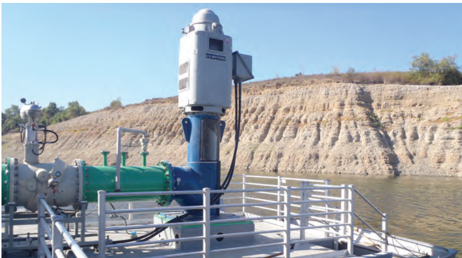
24" Tilting Disc Check Valve with Bottom Buffer and Top Mounted Hydraulic Cylinder and 2" Air Vacuum Valve at OCWD floating pump station.
