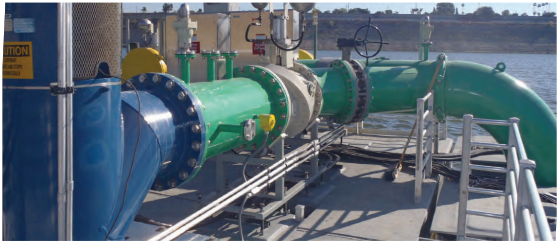
The GA Butterfly, Check, and Air Vacuum Valves installed on the floating pump station.
